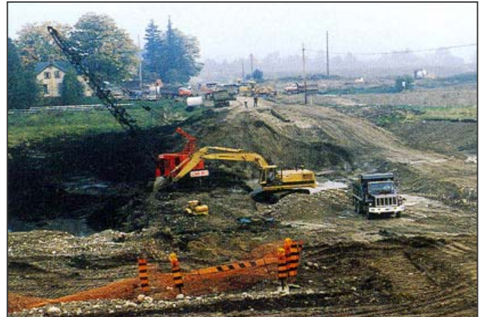
Photograph B2 - Excavation of a peat bog near the intersection of Fountain Street and Maple Grove Road.
