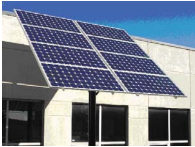
Solar Panel mounted on single pole in front of PLP's facility on Bishop Street
