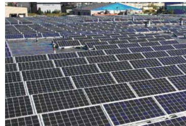
A 250kw rooftop installation on PLP's building
