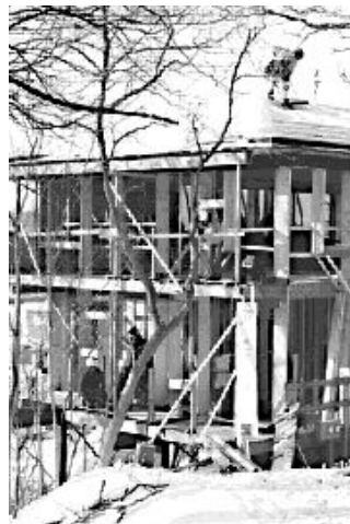
With the frame and roof in place, builders measured, kept the roof clear of snow and began installing insulation.
