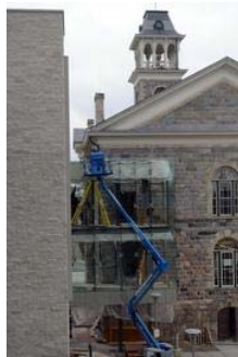
Construction workers are nearly done installing a glass bridge between the city's new office building and the rear corner of historic City Hall. This photo was taken a late September.
